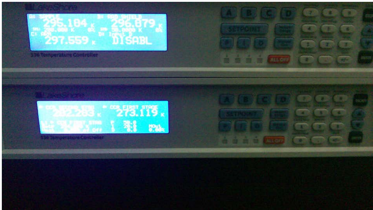
Fig. Temperature Controller Module
