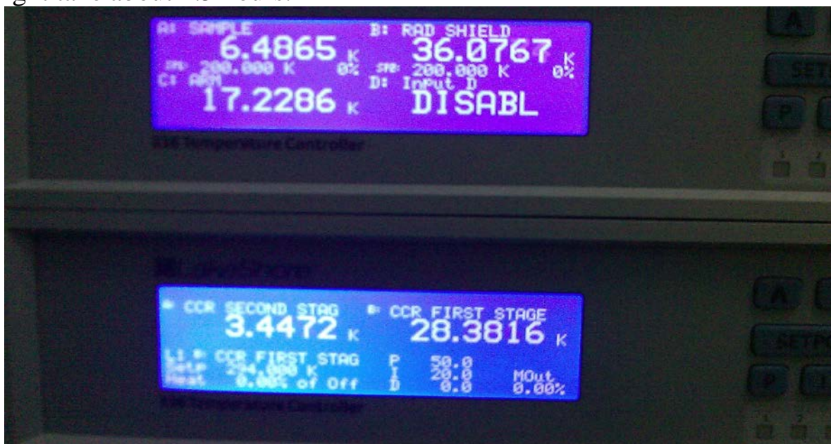
Fig. Temperature controller module
