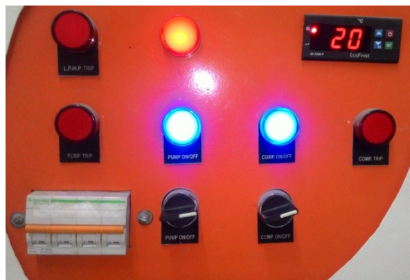
Fig. 3: Chiller at switch on condition
