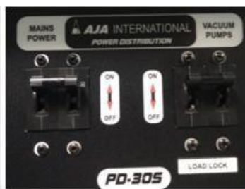
load lock ON
